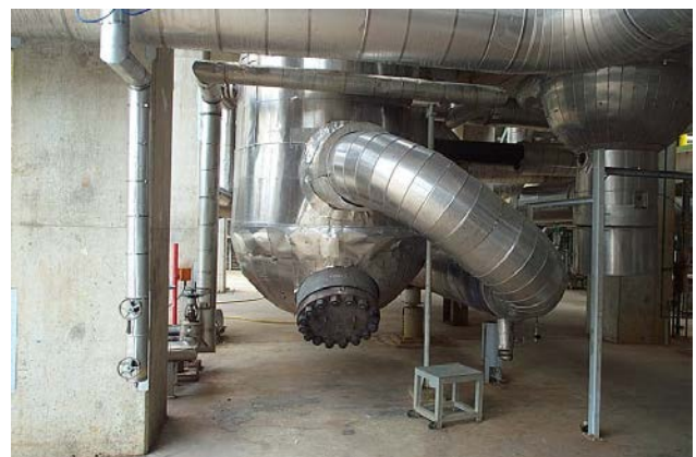
Figure 7. Channel section of superheater at KPA.
