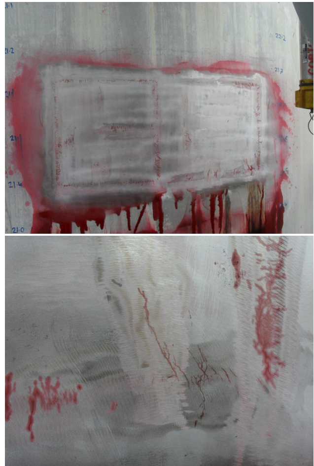
Figure 6. SCC under support plate at CSBP.
